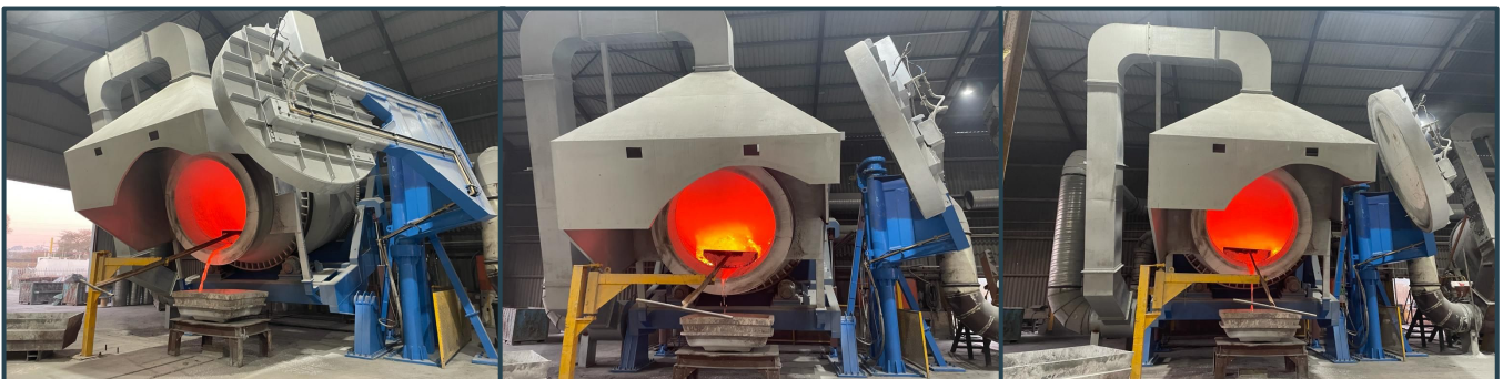
Furnace 4 at Alumicor commissioned in July 2021 increasing capacity by 250 tons per month.
